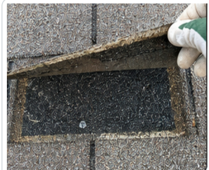
Lifted tab / compromised seal strip LIFTED TAB / FAILED SEAL
